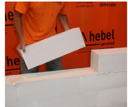
Figure 5D.8: Laying block by first setting backside down, then butting face of block is set into position
