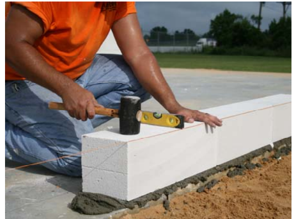
Figure 5D.4: Checking level and plumb, modify by tapping Hebel AAC block with rubber mallet
